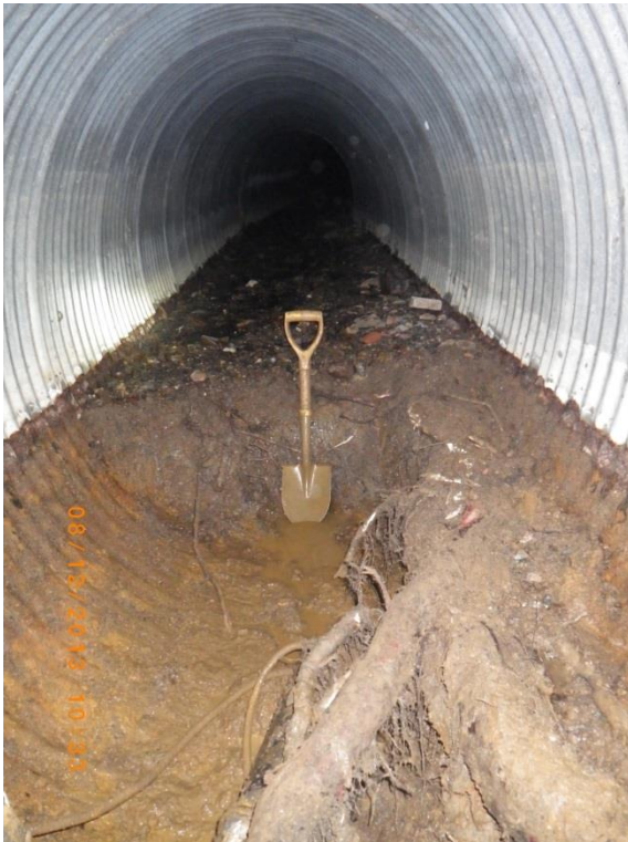
Pipe 30% full of debris and roots
