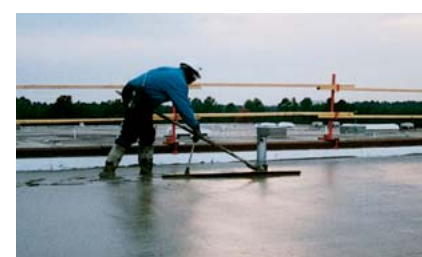
▲ Siplast Lightweight Insulating Concrete is screeded to a smooth, durable, monolithic surface ideal for roofing application.
