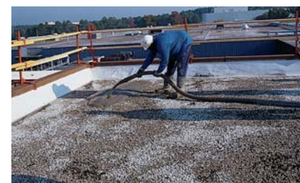
▲ On this reroofing project, a thin slurry coat of lightweight insulating concrete is poured in place, correcting substrate irregularities and bonding the Insulperm Insulation Board to the substrate.
