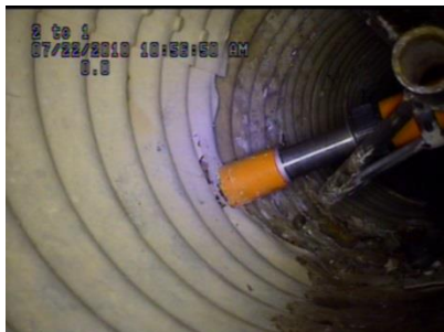
Snag-jack compresses tear points in the host pipe in preparation for the lining process
