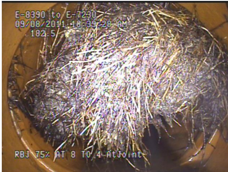
Existing problem identified
