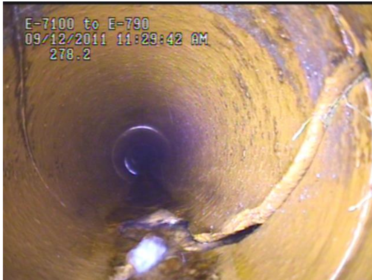
Existing problem identified
