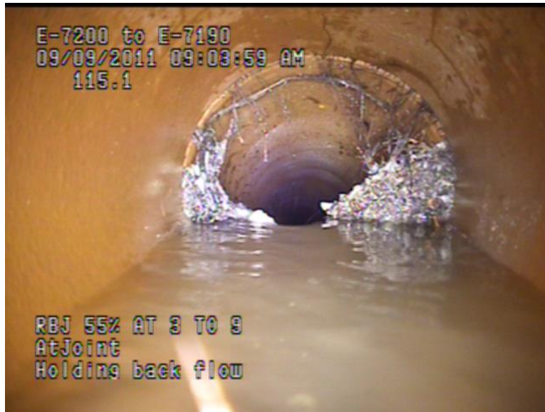
Existing problem identified
