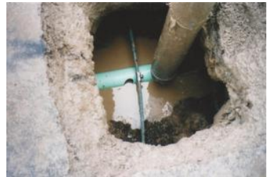
Hole discovered in sewer main caused by ruptured water main.
